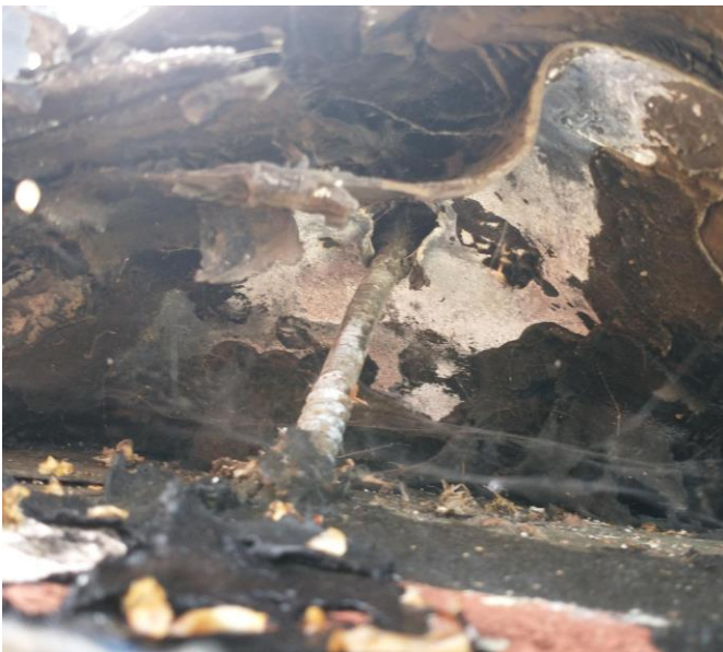
Guy wire anchor pulling out of roof.
