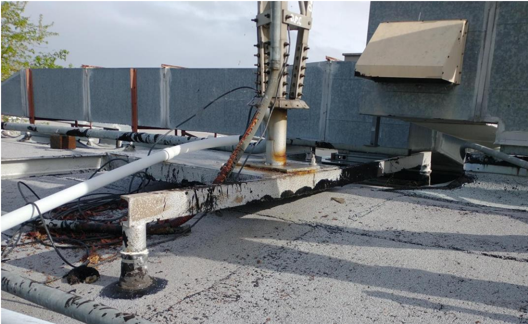
Deflection in tower support mounting frame
