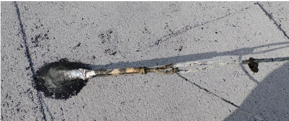
Non-Accessible turnbuckle and single cable clamp.
