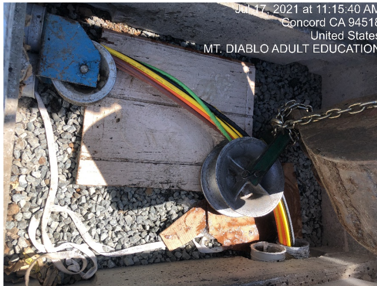
Pt B pullbox (new) with new 500 mcm cables
