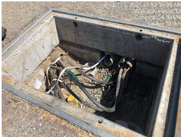
Existing pull box, conduit, and 500 MCM's (damaged)
