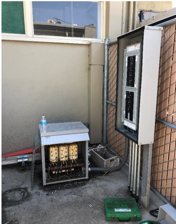
Panel LC and transformer (tied in)
